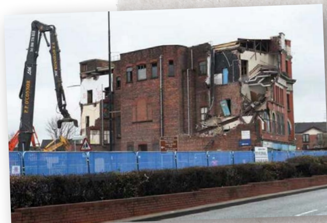
The demolition of Salford Central URC church. Photo reproduced from Manchester Evening News .
